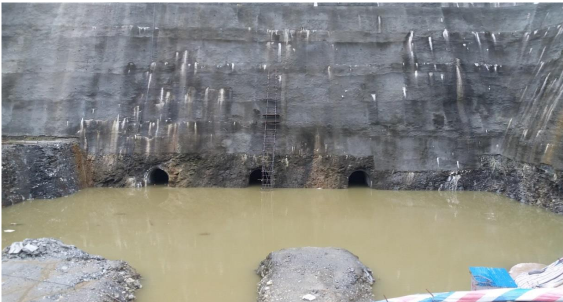
Plate 4.5: Water inundation at outlet of tri-furcation tunnel in PH Site
