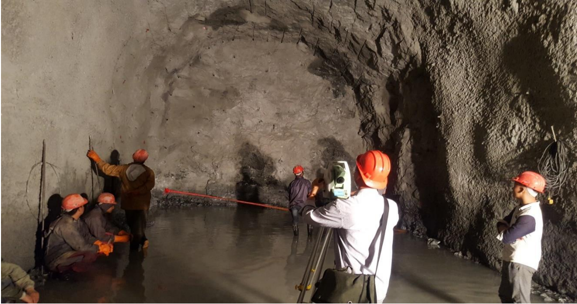
Plate 4.4: Water inundation inside HRT
