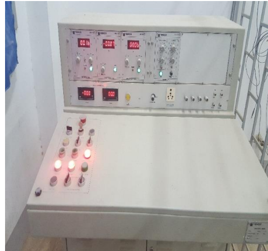
Figure 3: HV 9103 control desk includes measuring instruments and trigger device.
