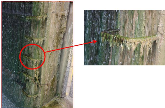
Figure 3: Inadequate application of a biocide (residual Chlorine in water= 1 ppm) without a proper biofilm thickening management (Reza Javaherdashti's Personal Collection). Biofilm developed on the concrete wall of the cooling tower (Left) and its magnified view (Right).
