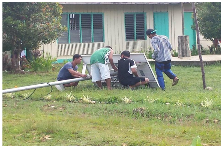
Plate No. 5: The installation of solar panel, photo taken last 2015 (Photo courtesy by Cherry Abne-Bruzon)
