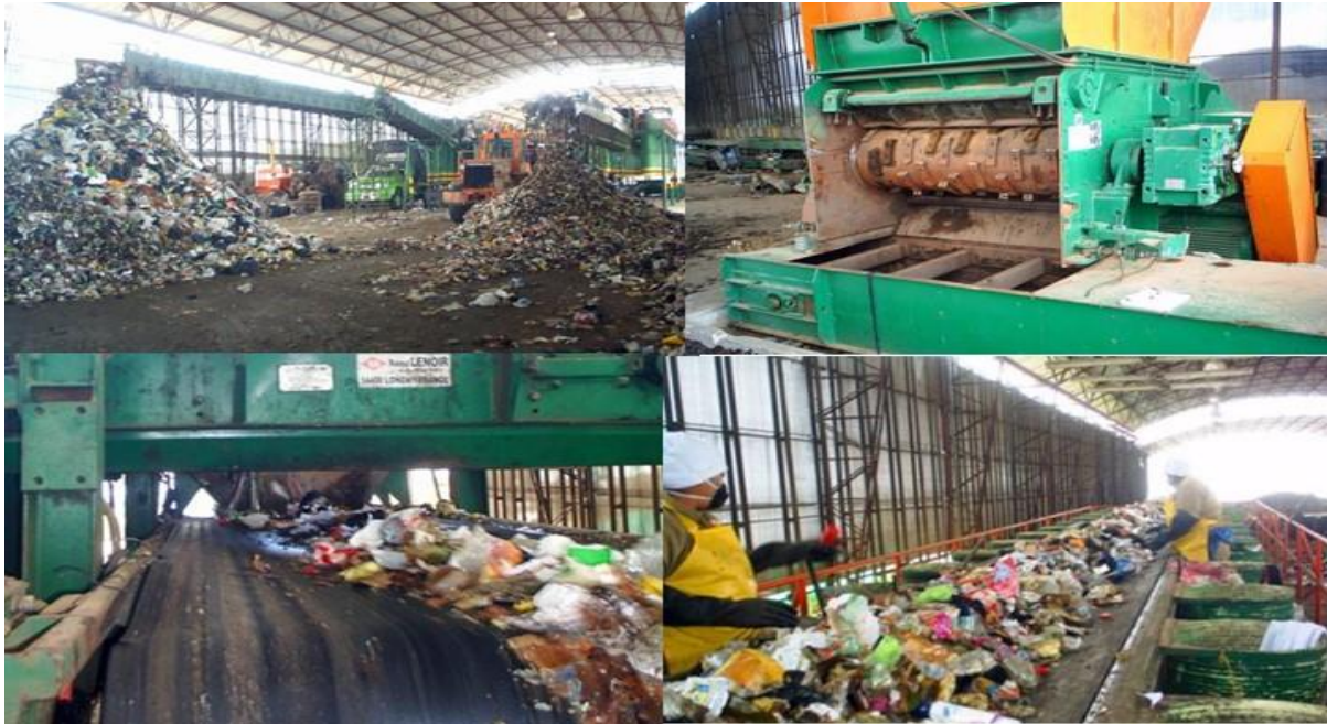
Figure 4: Collage of photographs showing aspects of the failed separation and recovery plant installed at El Guacal landfill site, now closed, (taken from a study done by the author)
