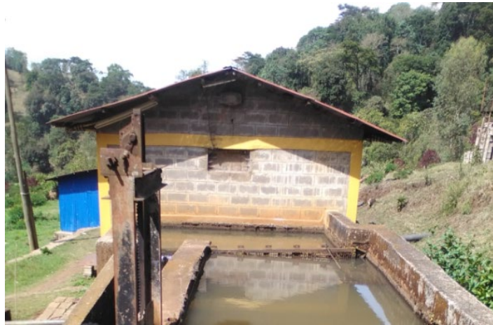
Figure 4: Forebay tank of the plant
