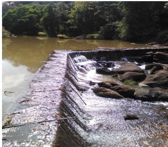
Figure 3: Weir of the plant
