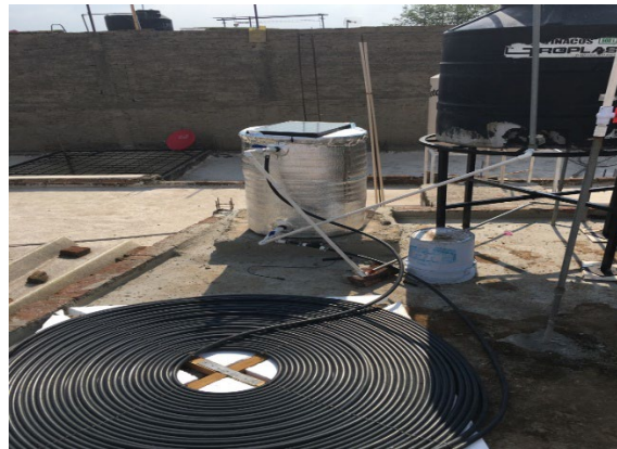
Figure 5 Solar Water Heaters
