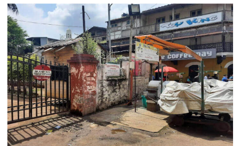
Figure 6c The Pyaav Currently Serves as a Platform to Stack Dustbins and Empty Water Buckets.
