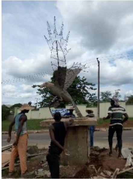
Plate 4 Gradual Buildup and Application of Mortar on the Constructed Armature Dimension: 275 Cm Diameter X 244 Cm High Medium: Cement, Sand, Mild Steel Rods, Chicken Wire and Binding Wire Year: 2021 Source: Ephraim Ugochukwu
