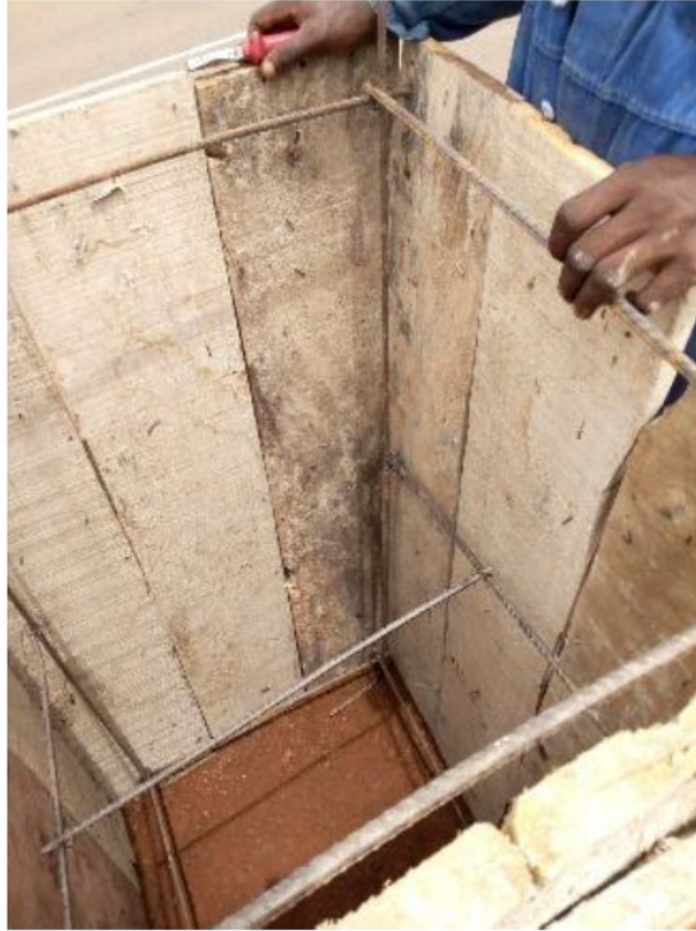
Plate 3 Armature Construction Dimension: 275 Cm Diameter X 244 Cm High Medium: Plywood, Metal Rods and Binding Wire Year: 2021 Source: Ephraim Ugochukwu
