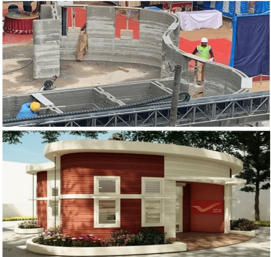
Figure 19 The Above Image Shows the 3D Printing Construction at Work Abraham (2023) , The Construction is Undertaken by the L&T Company Prasad (2023)
