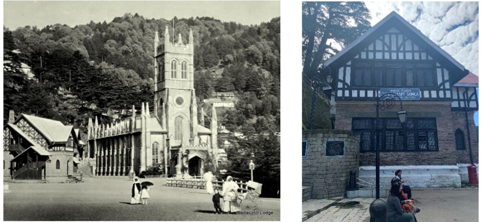
Figure 5 Façade of the State Library, Shimla with the Front Flight of Wooden Dog Leg Stairs Removed and Treated with the White Plastered Band at the Base on all Sides to Cover the Damp Surface.
